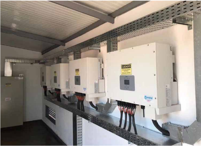
Brazil ▶ Inverter: SUN-80K-G Capacity: 320kW
